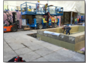
Example of a lift at a commercial job site
