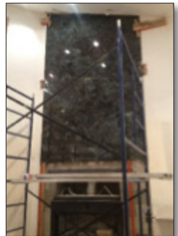
Example of a residential installation scaffold
